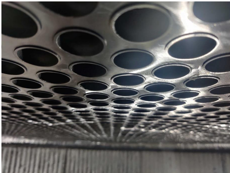
FIGURE 11: ALL THE TTS WELDS ARE REMOVED, THE TUBESHEET IS POLISHED AND THE TUBES START TO SLIDE DOWN WHILE THE CHANNEL IS LIFTED
